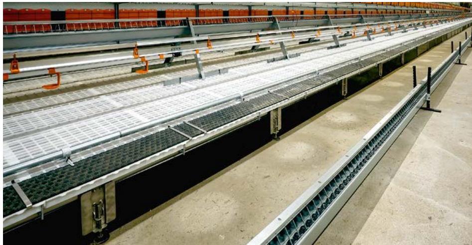
Winding manure removal system below the slat level with a jump height of just 280 mm
